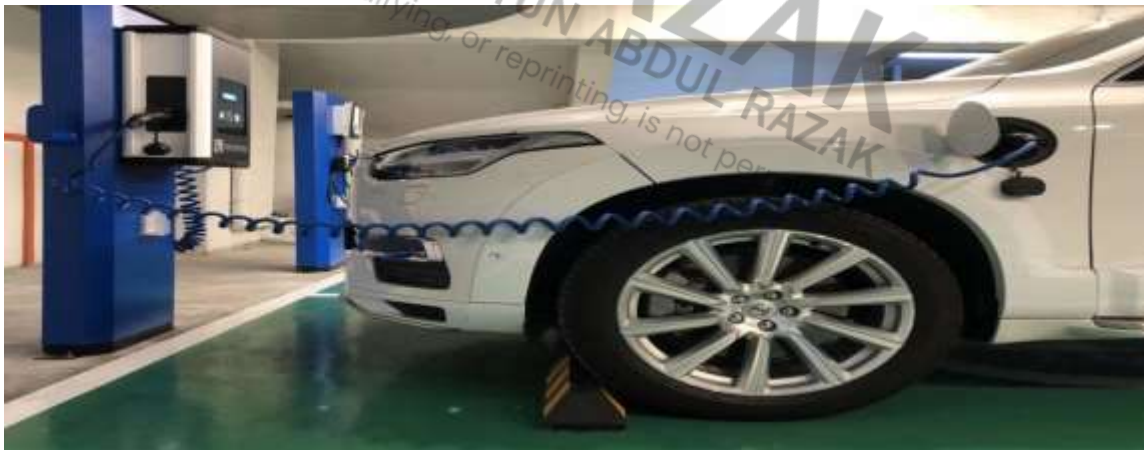
Figure 38. EV & PHEV Charging Station
